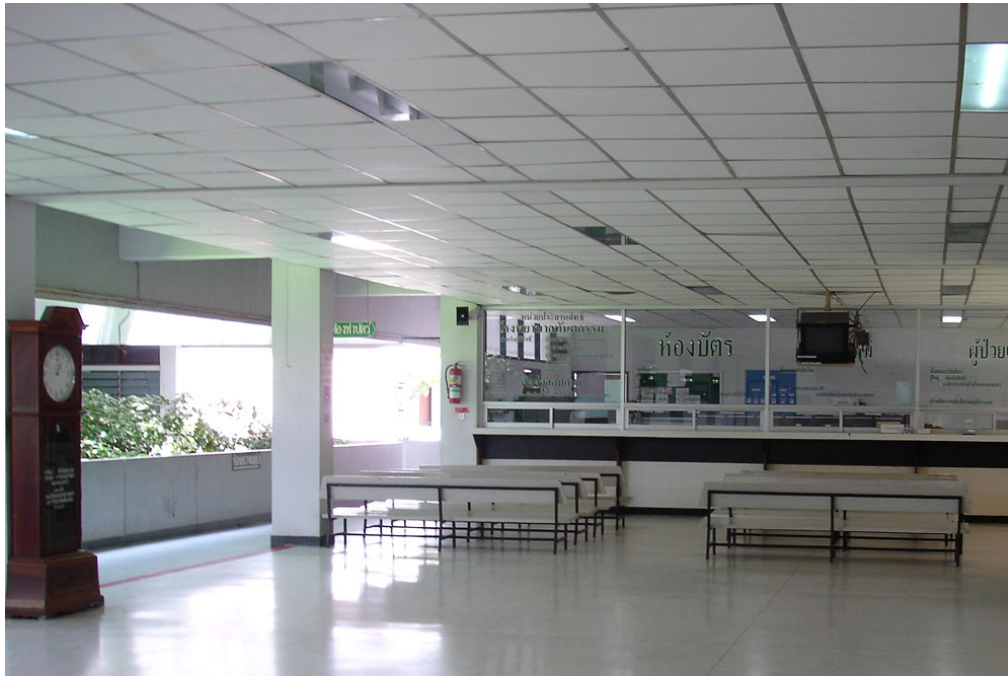
Figure 30: Gypsum board ceiling in Thailand normally installed with aluminum frame
