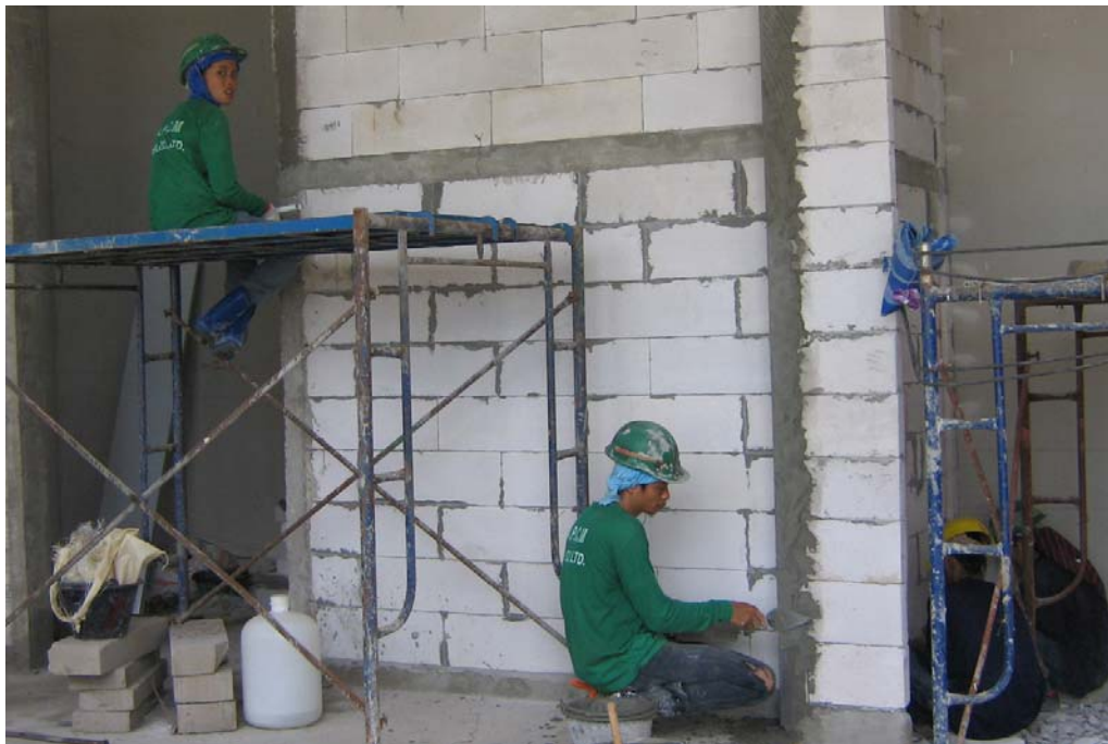
Figure 23: AAC construction – the mortar between each block is thinner than in other masonry materials
